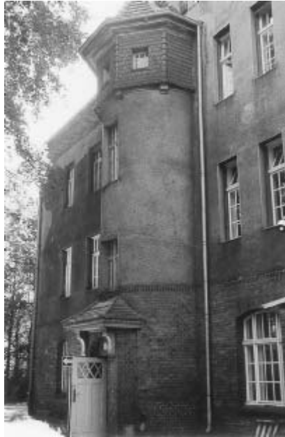
13.7 Landeslinik Eberswalde. Haus für ruhige Frauen, No.3. Built in 1905. Photograph by J. P. Boudreau, 2000.
