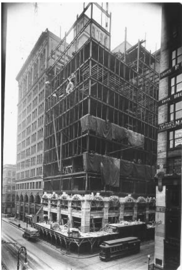
7.1 John Wanamaker Department Store, under construction, at Broadway between Eighth and Ninth Streets, ca. 1923. Photograph. New York Public Library.
